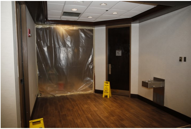
We got a look at the work being done at Embassy Suites.
